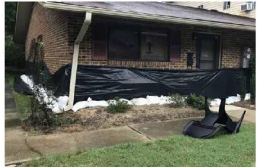
[23] A combination of different temporary measures can be an effective short-term solution to flooding. In this case, a building wrap of waterproof fabric is anchored by sandbags. Photo: Chapelhorn.com
