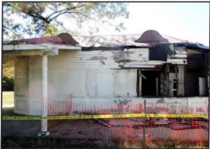
Figure 112. Concession Stand with Hurricane Isabel and other weather damage (taken in 2013).
